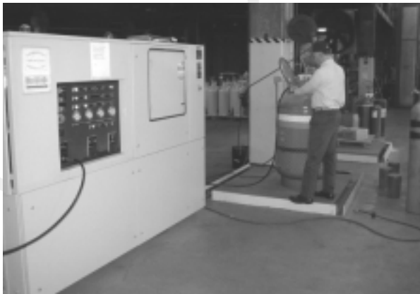
Technician connecting hose to a halon storage cylinder from a halon recycling unit operated in accordance with NFPA standards. EPA regulations prohibit disposal of halon except by sending it for recycling to a recycler operating in accordance with NFPA standards – or by arranging for its destruction via approved processes. Photo courtesy of U.S. DOD/DLA ODS Reserve.
